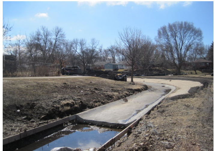
Construction on this new drainage ditch was started last fall and was never completed because of the weather. The old ditch is being replaced because of broken-up concrete not allowing water to drain.
