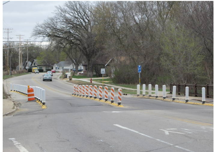
Pictured above is the Milwaukee St. bridge at the Fair Oaks intersection. It will be closed to traffic around July 1st to about the end of October for rebuilding.
