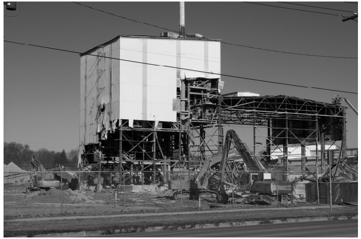
The major section of Royster-Clark has come down. By the time this newsletter is printed, the section pictured will be gone. The demo crew was fortunate to have the weather cooperate.
