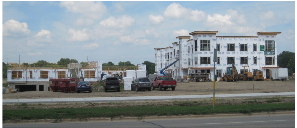
Pictured above shows the progress of Stonehouse/Moving-Out's buildings. The building on the right has reached it's height and the one on the left will catch up. Soon the other structures will start popping up.
