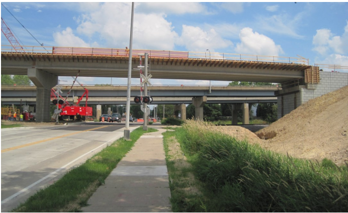
Pictured above is a partial view of the Cottage Grove Road Highway 51 Overpass. It is designed to improve 51 south traffic access to Cottage Grove Road and Cottage Grove Road traffic access to 51 heading south.
