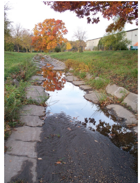
Picture of the drain ditch behind Woodman’s grocery. Concrete is all broken up and in chunks, along with accumulation of soil and standing water that does not drain as intended.
